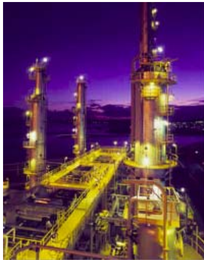
Fluid catalytic cracking unit
