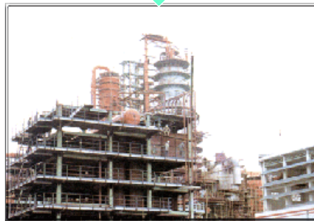
Solids waste incinerator
